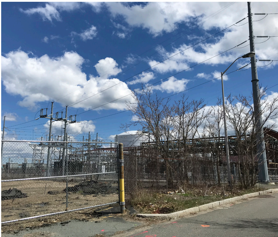
National Grid Substation
